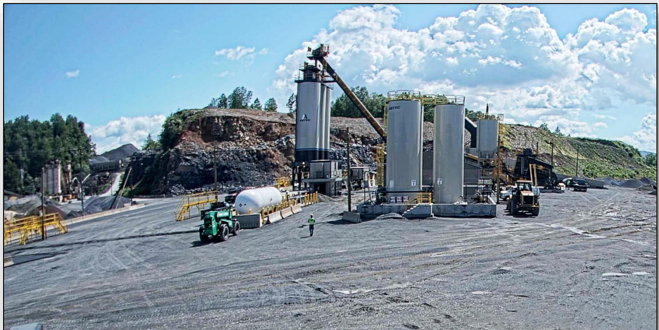
A "live" Earthcam photo of Easton Asphalt as captured on June 9, 2022, or date of this Press Release showing current construction progress of the facility.
