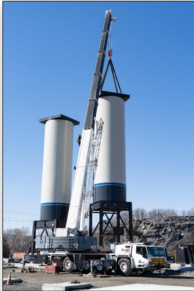
H&K's new Easton Asphalt facility goes vertical with placement of the second 300-Ton silo.
